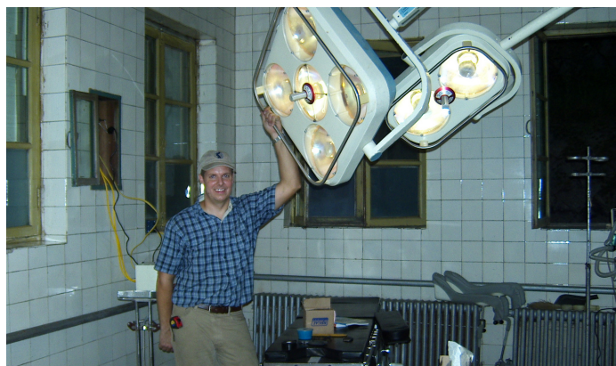
Newly installed operating room lights.
