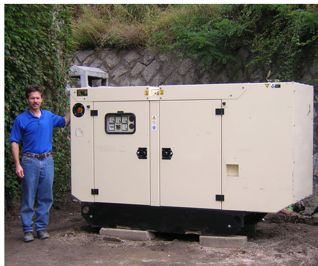
Newly installed generator.
