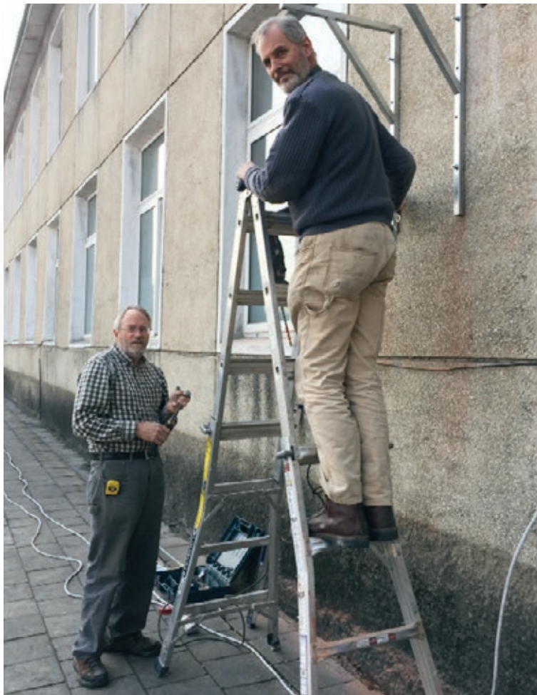
Tom Linton and Rob Robinson install wiring at the Pyongyang #2 Hepatitis Hospital
