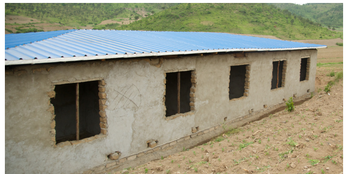
A nearly completed roof has been installed on a new patient ward under construction at Hwangju TB Sanitarium.
