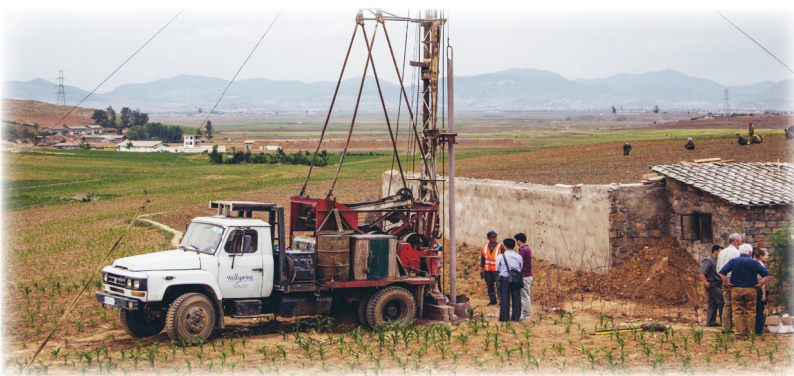
Well being repaired by Wellspring drilling rig at Sariwon #3 TB Rest Home.
